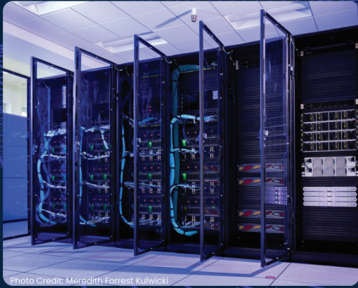
Supercomputing center of Empire AI, located at University at Buffalo.
