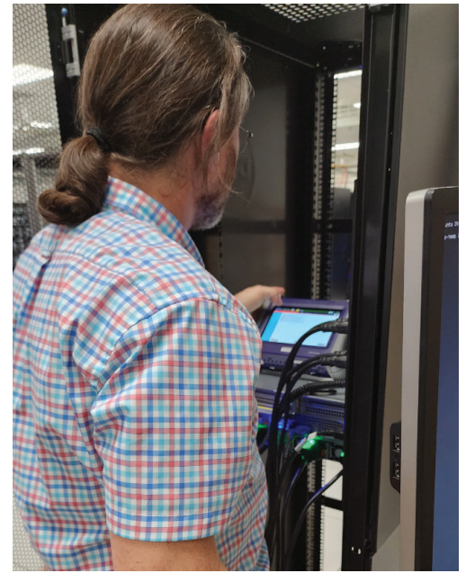
Bobby Clark, Network Engineer for ARE-ON, completes the testing of the GP-ENGINE node
